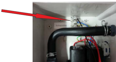
Connection Float Switch
